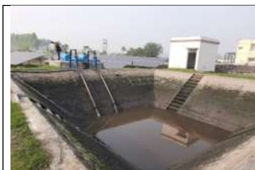
Photo 1. Solar Panel, TWW tank, Control Head
